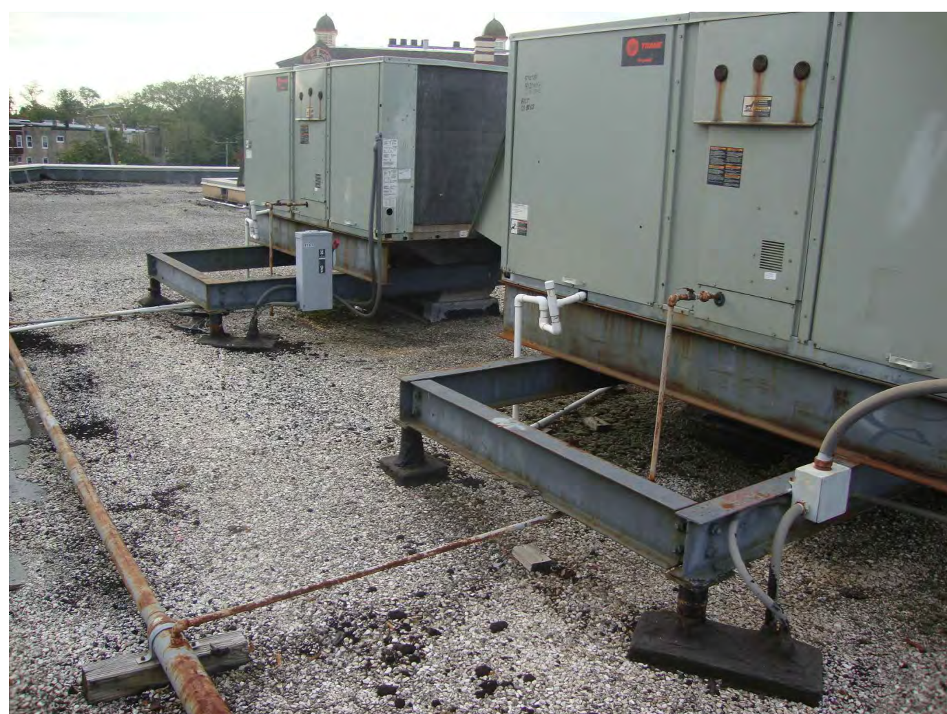
PHOTO # 21 - ROOF TOP UNIT ON DUNNAGE AND CONDUIT PENETRATION
