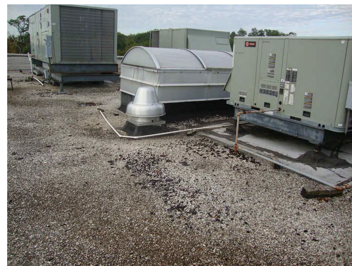
PHOTO # 23 - ROOFTOP EQUIPMENT
