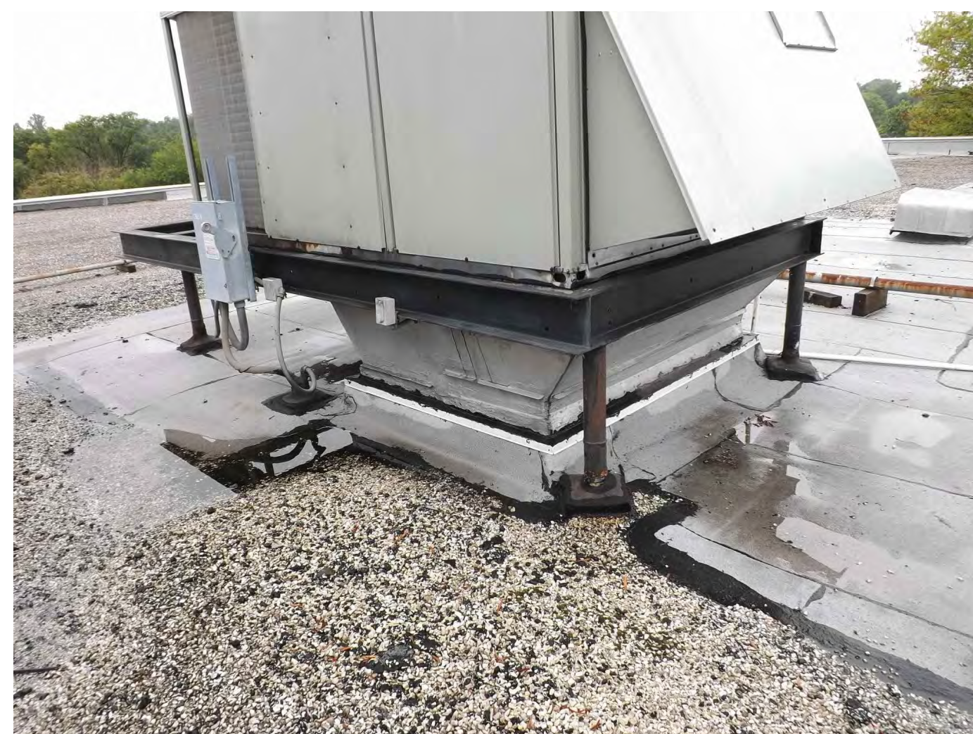
PHOTO # 34 - ROOF TOP UNIT ON DUNNAGE SUPPORTS
