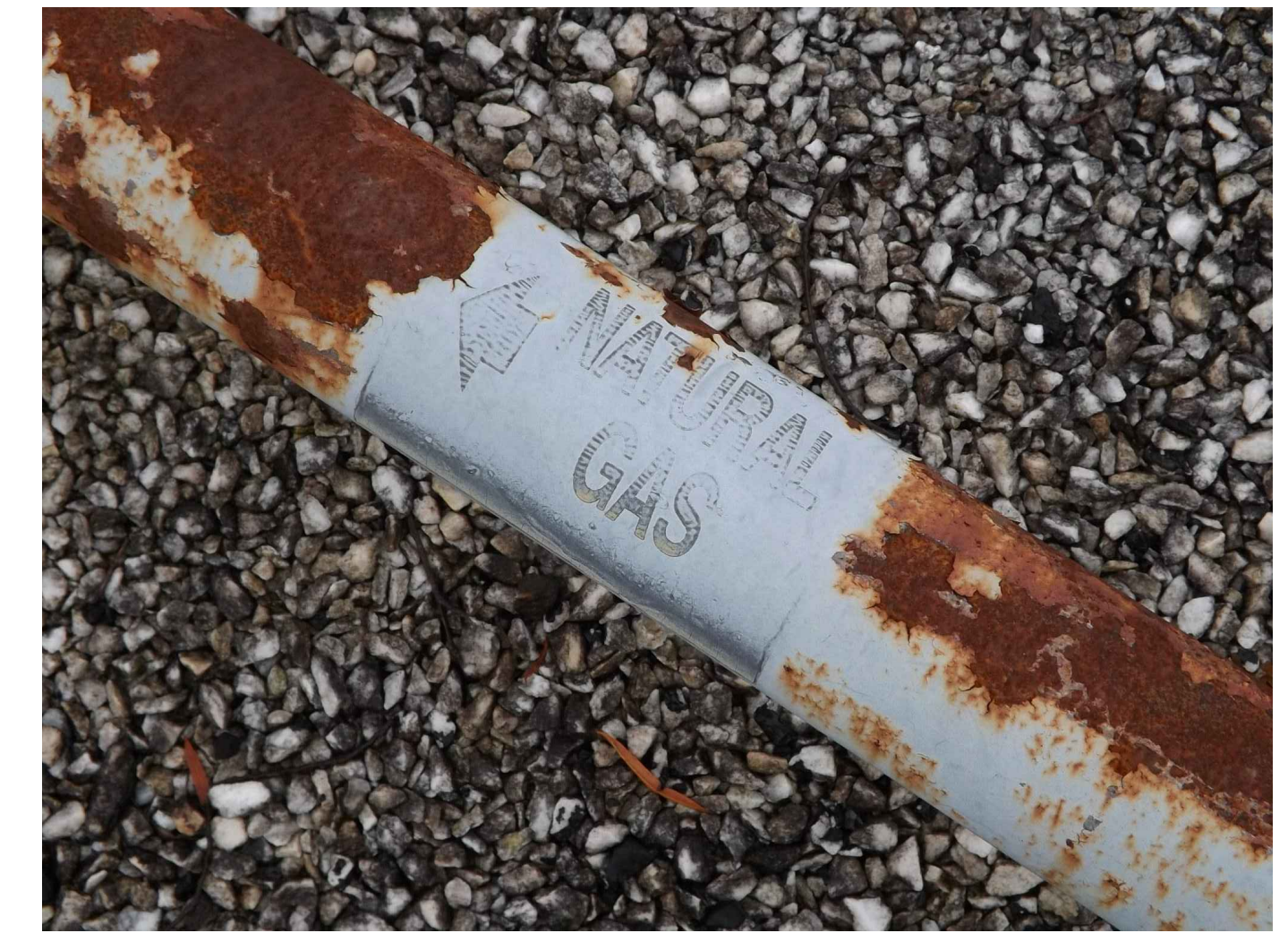
PHOTO # 32 - GAS LINE AT MAIN ROOF
