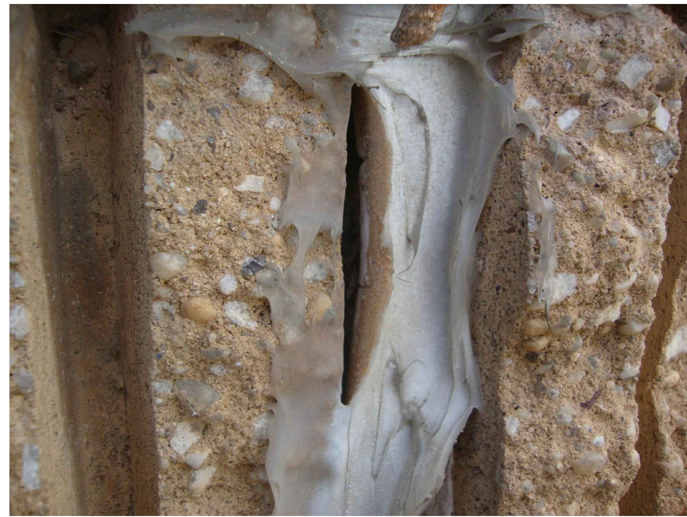
PHOTO # 30 - OPEN SEALANT JOINT
