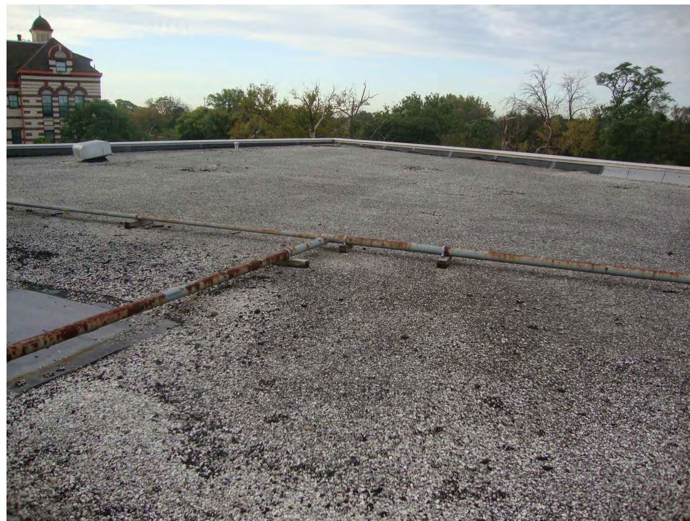
PHOTO # 17 - GAS LINE AT MAIN ROOF
